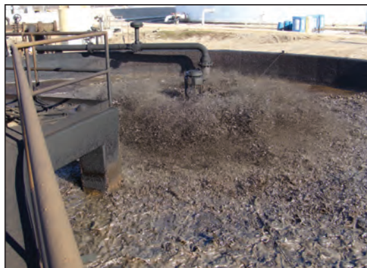
FIGURE 1. In this step of the biological wastewater treatment, the activated sludge is aerated
