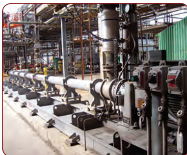
SP1000 pump installation at Texas refinery for wash water service
